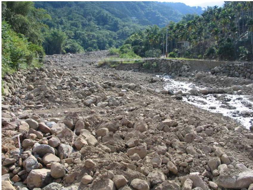
Figure 3. A project using ecological engineering methods that failed due to Typhoon Mindulle
