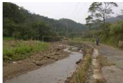
♦ Improved Channel after flood events in year 2004
